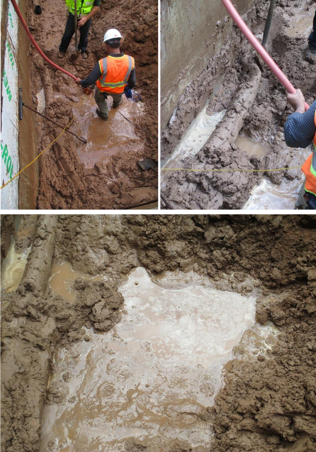
Figure 101. Bottom of the excavation near the drain tile on the south abutment after pumping out the ponded water
