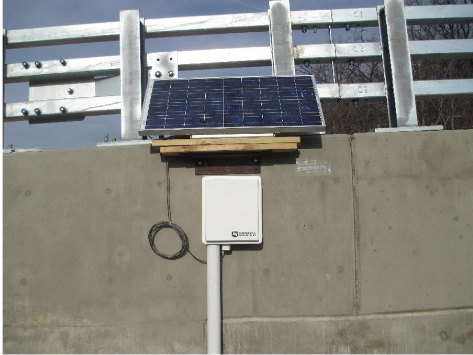
Figure 40. Sealed enclosure and solar panel used for the DAQ system
