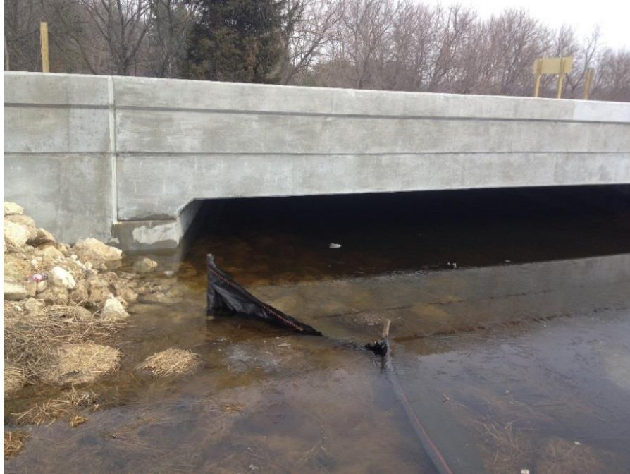
Figure 91. Water ponding on April 7, 2014
