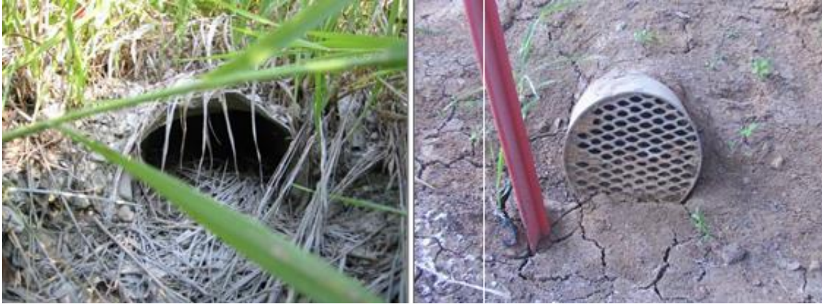
Figure 1. Examples of clogged end drains at I-80 bridge over McPearson Avenue (left) and the bridge on US 218 over South Skunk River (right) (White et al. 2005)
