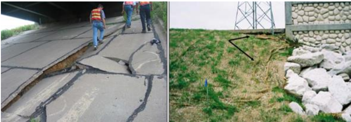
Figure 2. Examples of (left) severe damage of concrete slope protection due to erosion on I-380 bridge over Hwy 6 in Iowa (White et al. 2005), and (right) slope instability on West Beloit Road Bridge over Root River in Wisconsin (Helwany et al. 2007)
