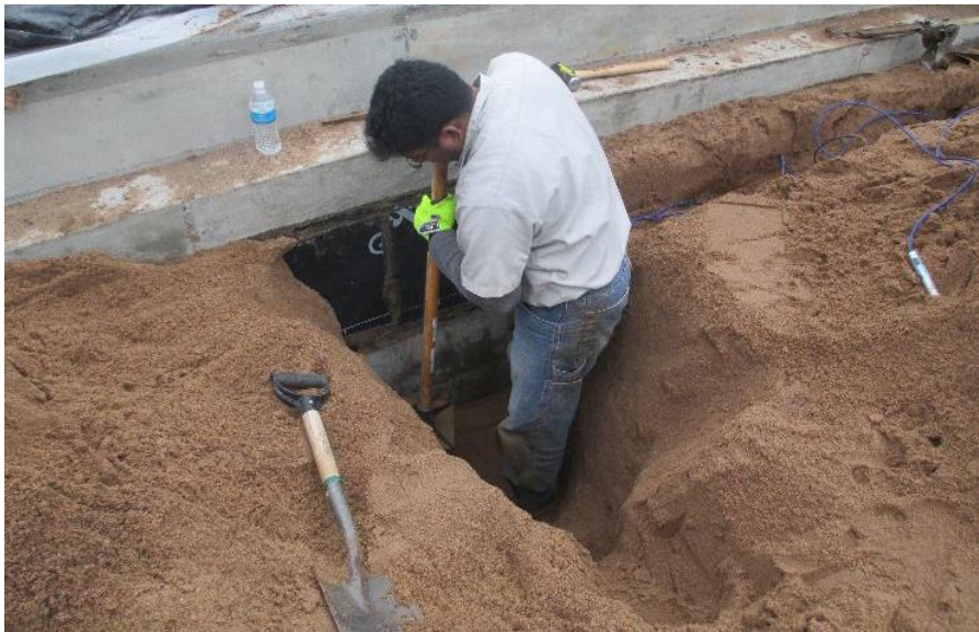
Figure 88. Compaction of backfill material in thin layers after installing PP and EPC sensors at multiple depths
