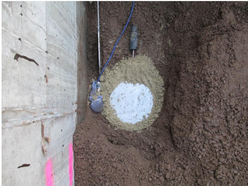
Figure 125. Vertical EPC and pore pressure sensor installation at Hobbles Creek Bridge
